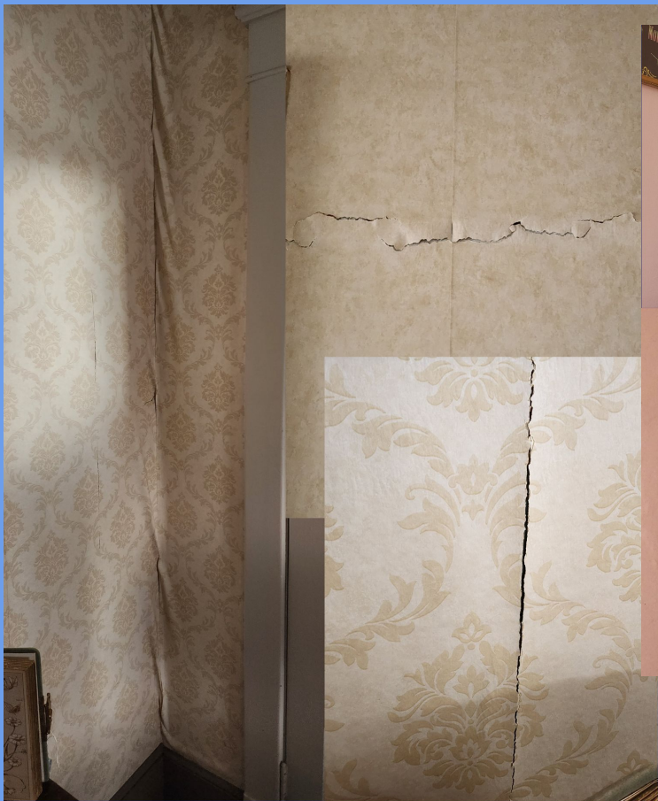
Damaged wallpaper in living room
