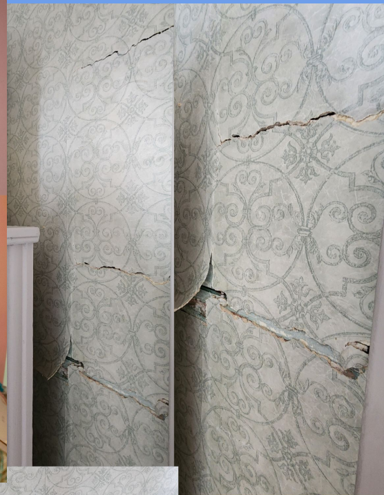
Damaged wallpaper in kitchen
