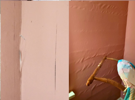
Damaged wallpaper in small room downstairs
